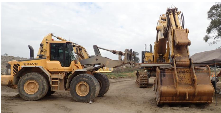
Figure 1 - Intended method to extract excavator pin
