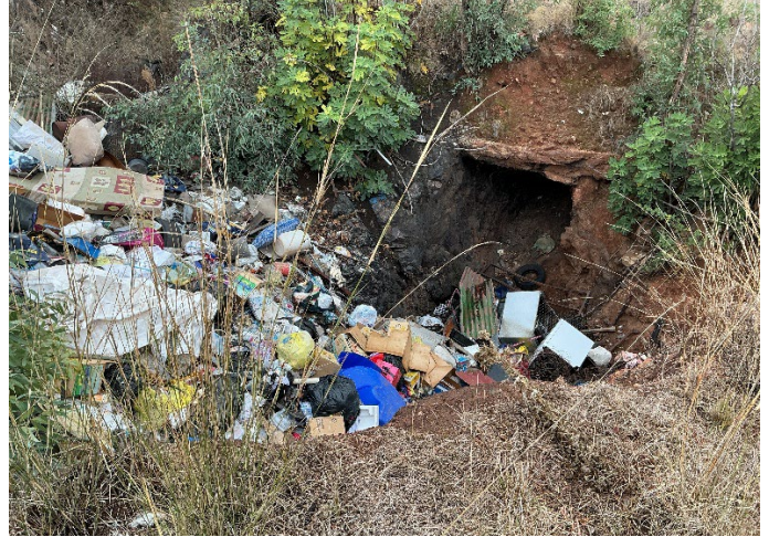
Figure 2: Waste dumped on junior adit
