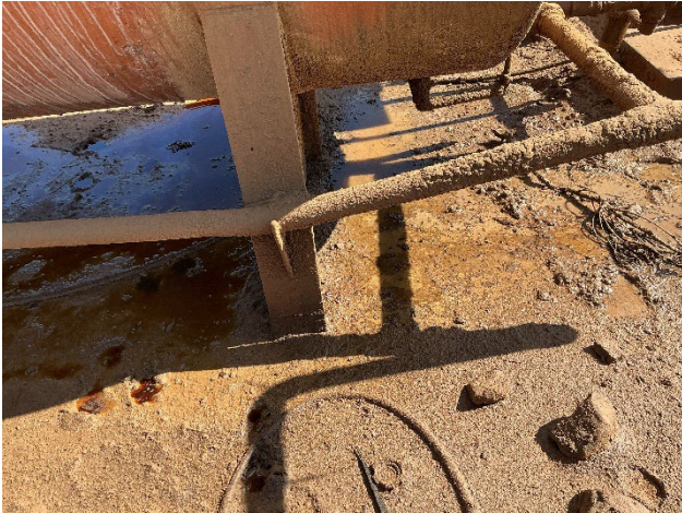
Figure 7: Diesel storage bund
