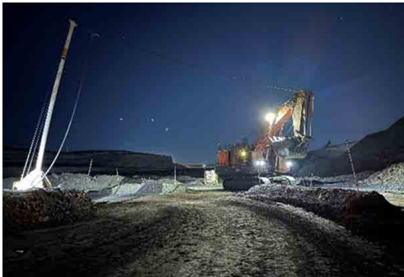
Picture 2. Excavator in contact with cable.
