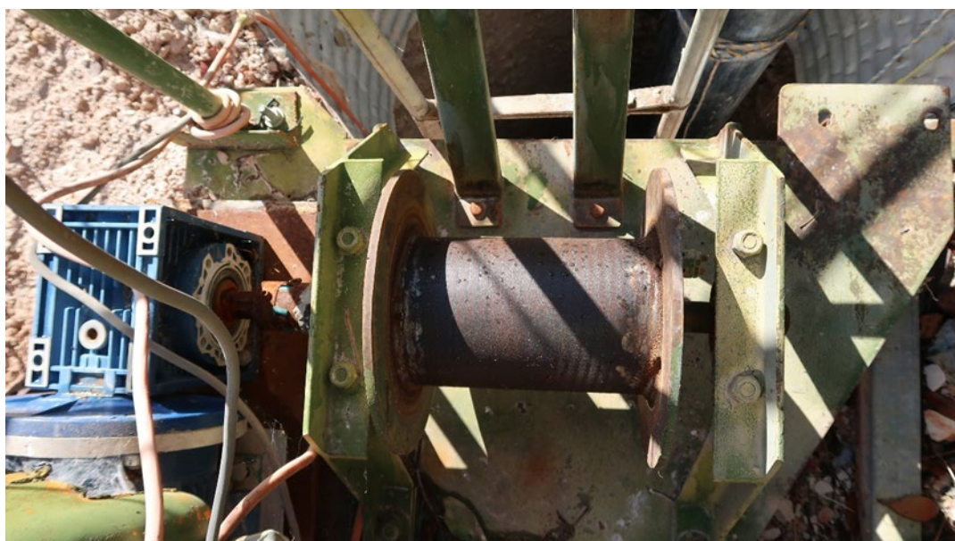
Figure 2: Cable from hoists drum was found completely unspooled
